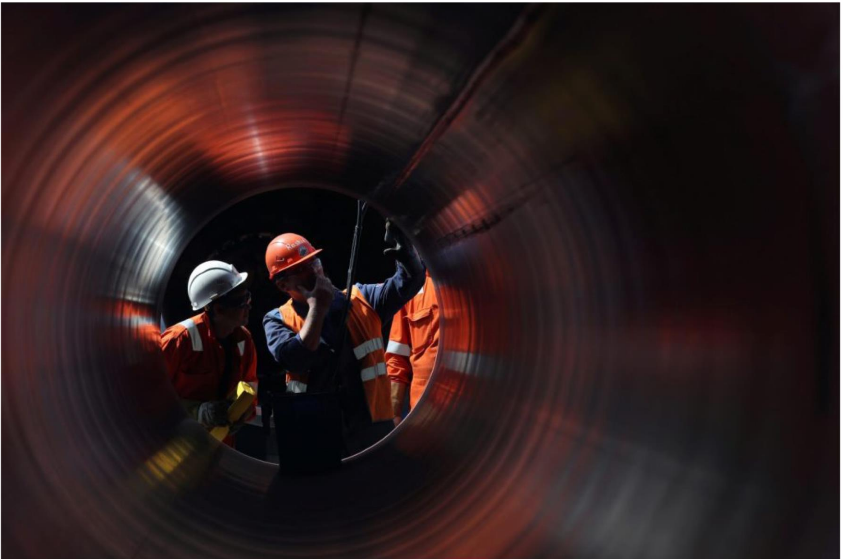
Workers are seen through a pipe at the construction site of the Nord Stream 2 gas pipeline, near the town of Kingisepp, Leningrad region, Russia, June 5, 2019. REUTERS/Anton Vaganov
