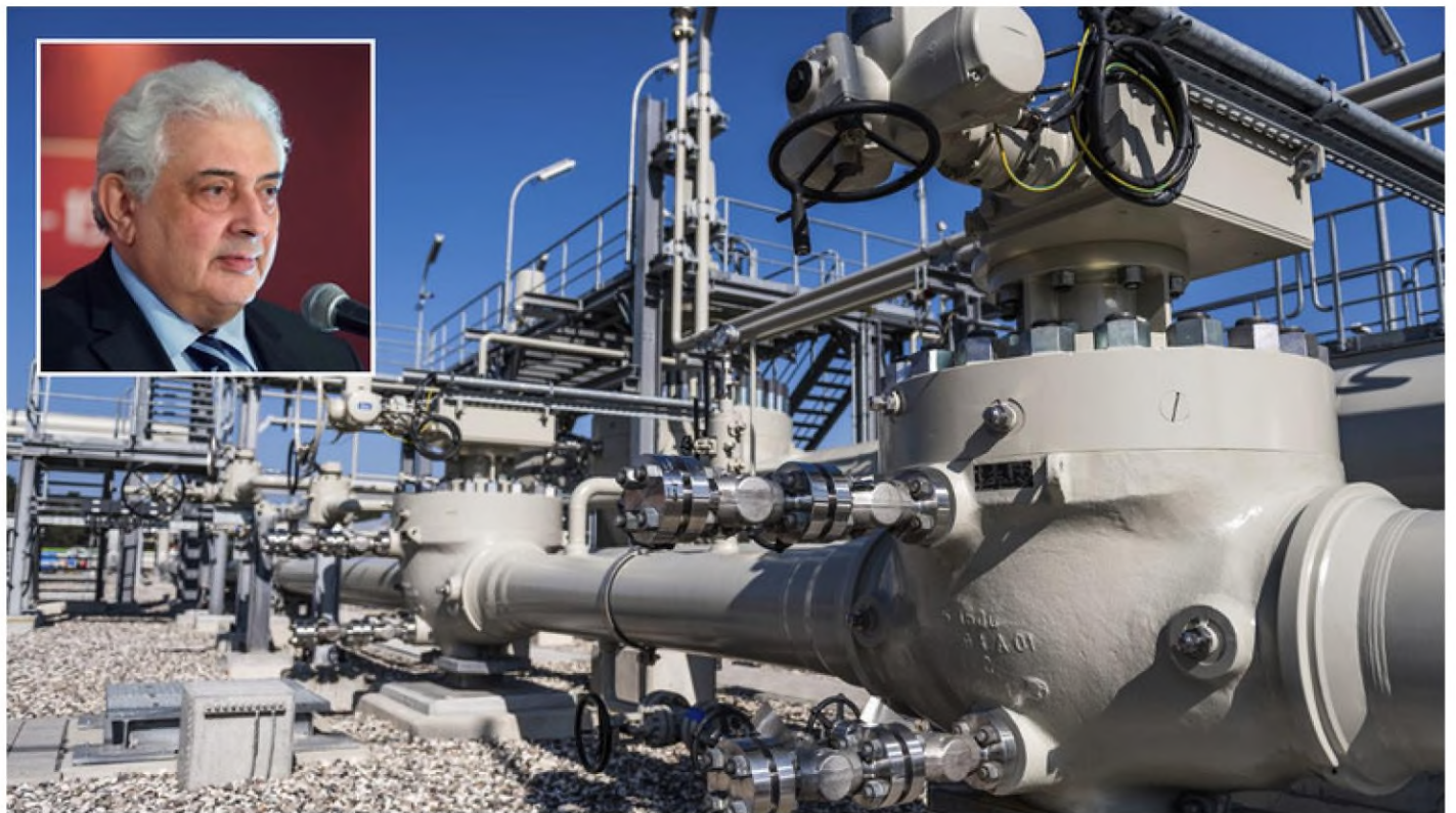
Piping systems and shut-off valves are pictured at the gas receiving station of the Nord Stream Baltic Sea pipeline, in Lubmin, Germany. © Sputnik / Dmitrij Leltschuk; (inset) Russian Ambassador to Germany Sergey Nechayev © Sputnik / Igor Zarembo
