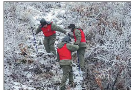
State Grid Wuhan employees do maintenance work in Hubei province. PROVIDED TO CHINA DAILY
