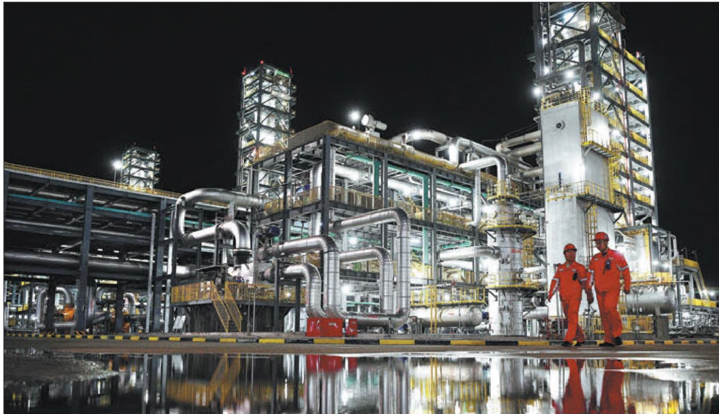
Technicians from China National Petroleum Corp conduct an inspection at a natural gas processing facility of Changqing oilfield in Yulin, Shaanxi province, in July. WANG PENG / XINHUA
