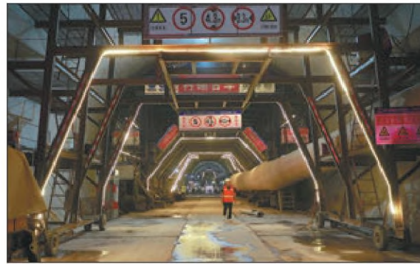
An employee of China Railway 24th Bureau Group Corp inspects a tunnel on the Jinhua-Jiande High-speed Railway project in Zhejiang province in September. PROVIDED TO CHINA DAILY
