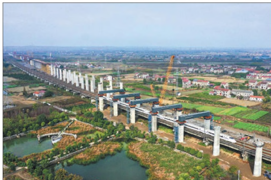
Right: A high-speed train crosses a new bridge in Jingzhou built from steel girders. Installation of the girders was completed in November. XU YUNHUA / FOR CHINA DAILY
