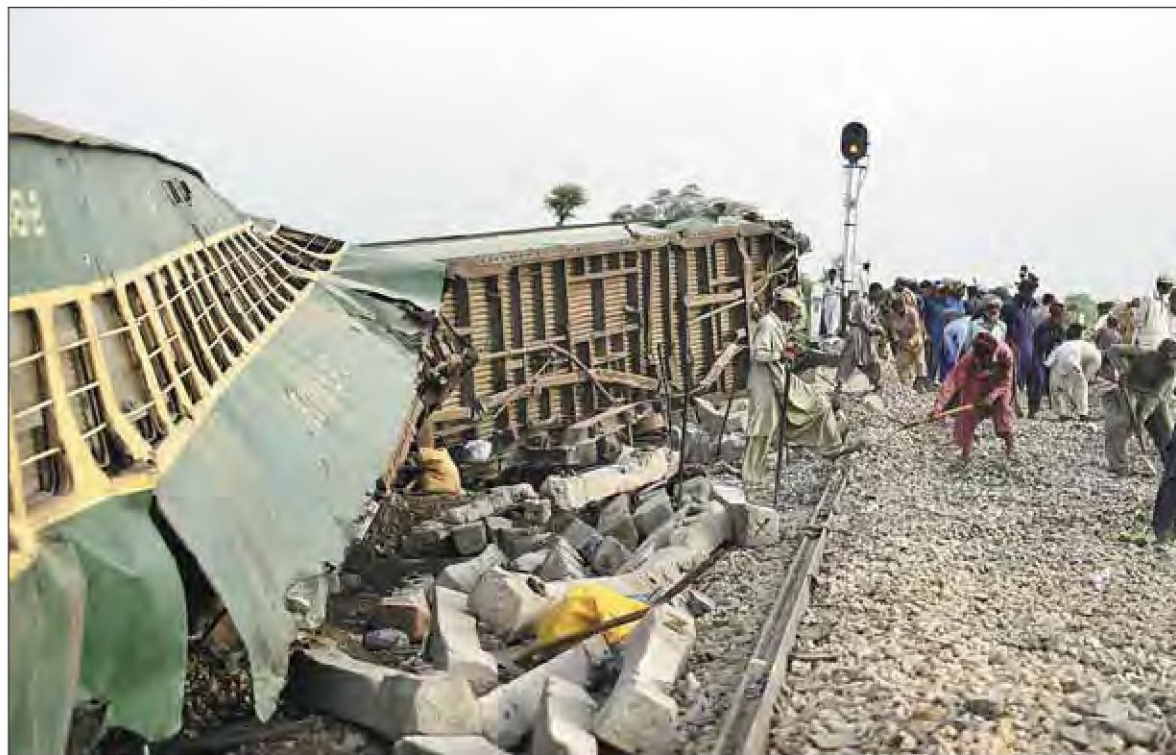
Railway workers repair tracks on Monday next to damaged carriages a day after a passenger train derailed in Nawabshah, Pakistan. The accident killed at least 34 people. ASIF HASSAN / AFP See story, page 5
