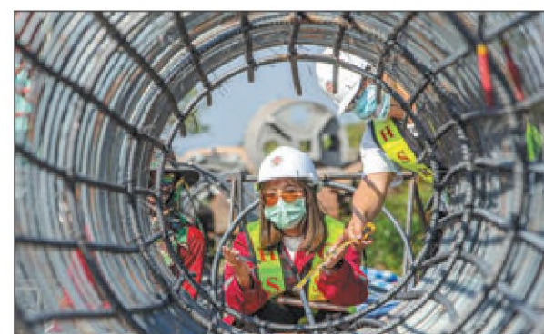
A girl works at a construction site of the China-Thailand railway in Nakhon Ratchasima Province, Thailand, on Feb 23. WANG TENG / XINHUA
