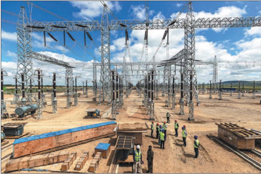
Visitors tour the 400-kV Konza substation in Konza, Kenya. XIE SONGXIN / CHINA DAILY
