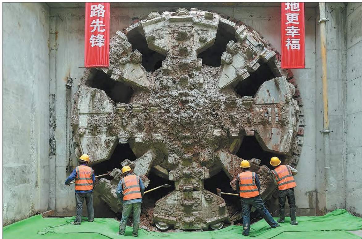
Workers ready a tunneling machine at a construction site of Hefei Metro in Anhui province in March. The urban rail project under construction is partly being built by China Railway 24th Bureau Group Corp Ltd. YUAN BING / FOR CHINA DAILY
