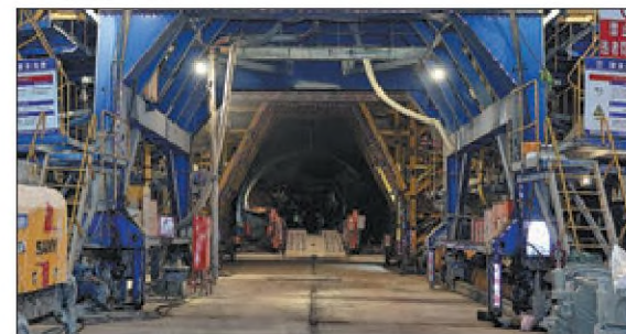
Construction site of the Fengzhen Tunnel on the Jining-Datong-Yuanping High-speed Railway in North China. The 290.1-kilometer railway, which is partly built by China Railway No 4 Engineering Group Co Ltd, aims to better link Shanxi province with the Inner Mongolia autonomous region. WANG SHUQUANG / FOR CHINA DAILY
