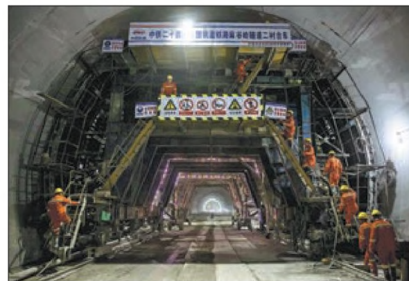
Construction workers of China Railway 24th Bureau Group Corp Ltd work at the Maguling Tunnel on the Hangzhou-Wenzhou High-speed Railway in Zhejiang province on April 3. JIANG HAN / XINHUA
