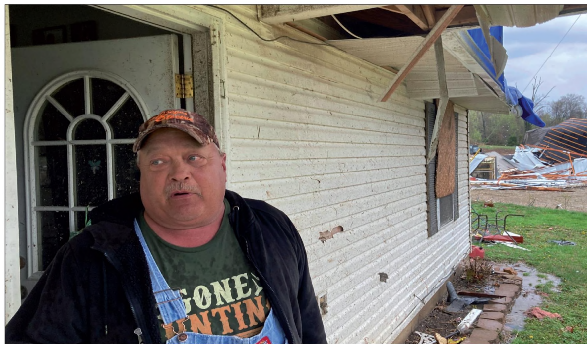
Keith Lincoln stands outside his damaged home in Glen Allen, Missouri, on Wednesday. A large tornado tore through southeastern Missouri before dawn on Wednesday, killing several people and causing widespread destruction. JIM SALTER / AP
