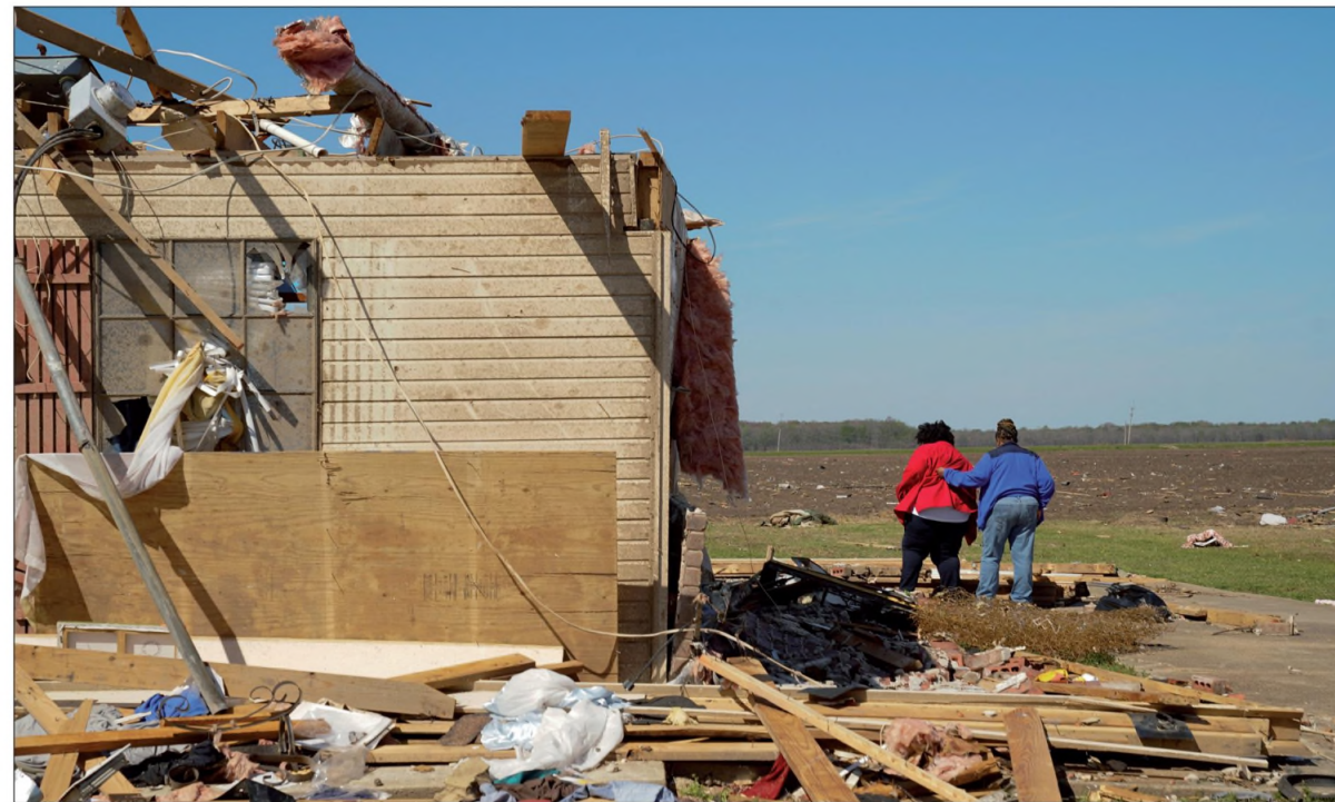
Chandra Wells, 47, and her sister Jennifer, 57, walk past the wreckage of Chandra's home after thunderstorms spawning high straight-line winds and tornadoes ripped across the state, in Rolling Fork, Mississippi, on Monday. At least 21 people were killed in the state. CHENEY ORR / REUTERS
