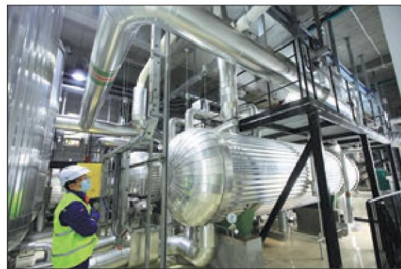
Steam generated from a reactor in Dalian, Liaoning province, is used as a source of heat. PROVIDED TO CHINA DAILY
