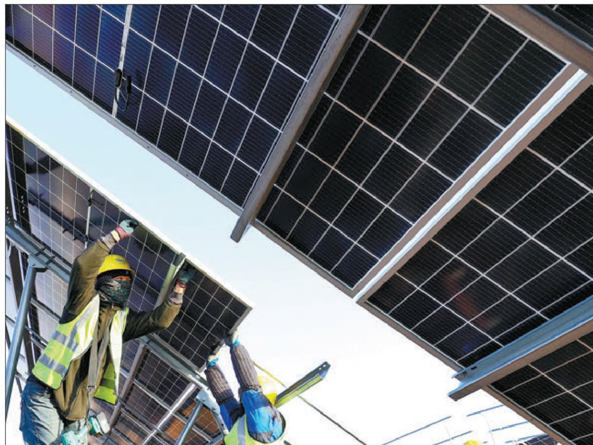
Technicians install photovoltaic panels at a solar power plant in Zhangye, Gansu province, in December. WANG JIANG / FOR CHINA DAILY
