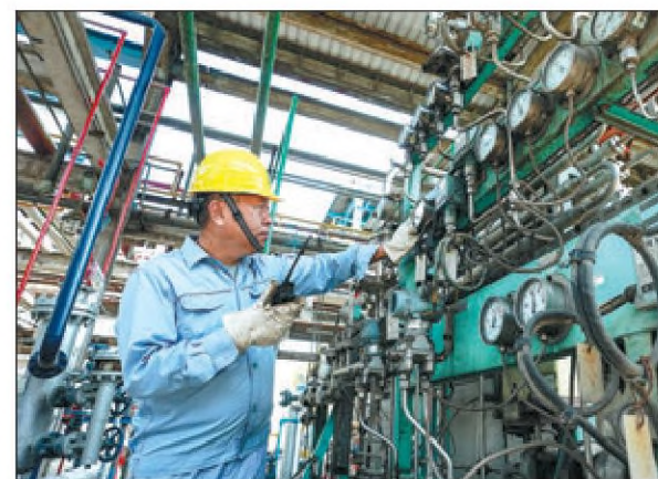
A Sinopec employee inspects refinery equipment in Huai'an, Jiangsu province, in August. ZHAO QIRUI / FOR CHINA DAILY
