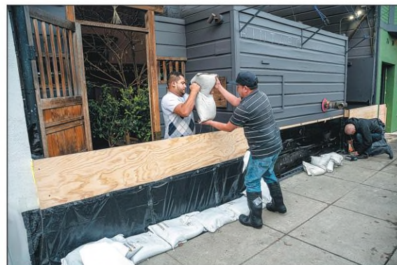
Workers build a flood protection barrier at the entrance to a business in San Francisco, California, on Tuesday. While California tries to clean up from floods and mudslides that killed at least one person over the weekend, the next in a series of atmospheric rivers is bearing down on the state later this week. VIA GETTY IMAGES
