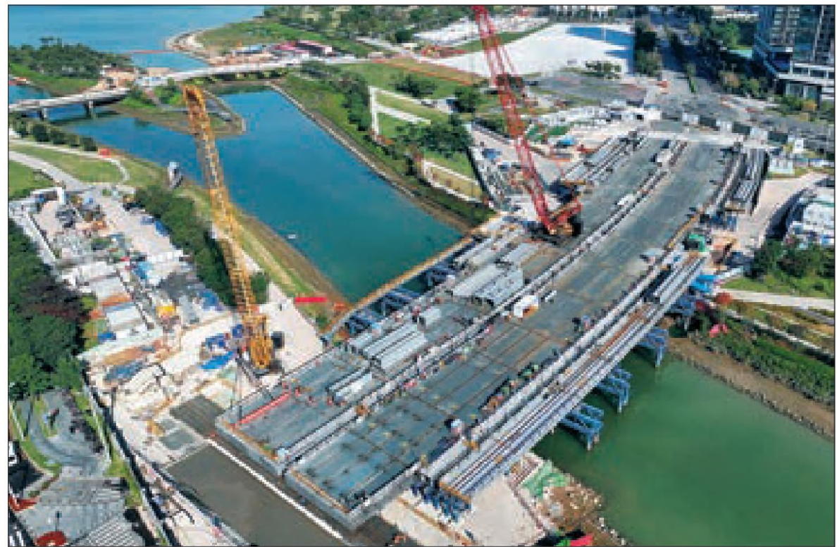
Construction workers are seen working at a bridge connecting project in Shenzhen, Guangdong province, on Wednesday. Builders from China Railway No 4 Engineering Group Co Ltd have fully connected the Guiwan River Bridge in Shenzhen, helping to perfect Qianhai area's transport. Officials in Shenzhen said this will aid the internationalization of its Qianhai Shenzhen-Hong Kong Modern Service Industrial Cooperation Zone. PROVIDED TO CHINA DAILY
