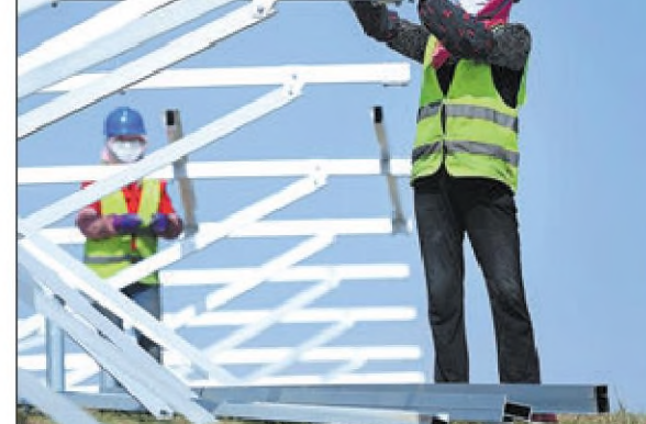
Center: Workers assemble solar panels to expand the use of clean energy along the river in Qinghai province. ZHANG LONG / XINHUA
