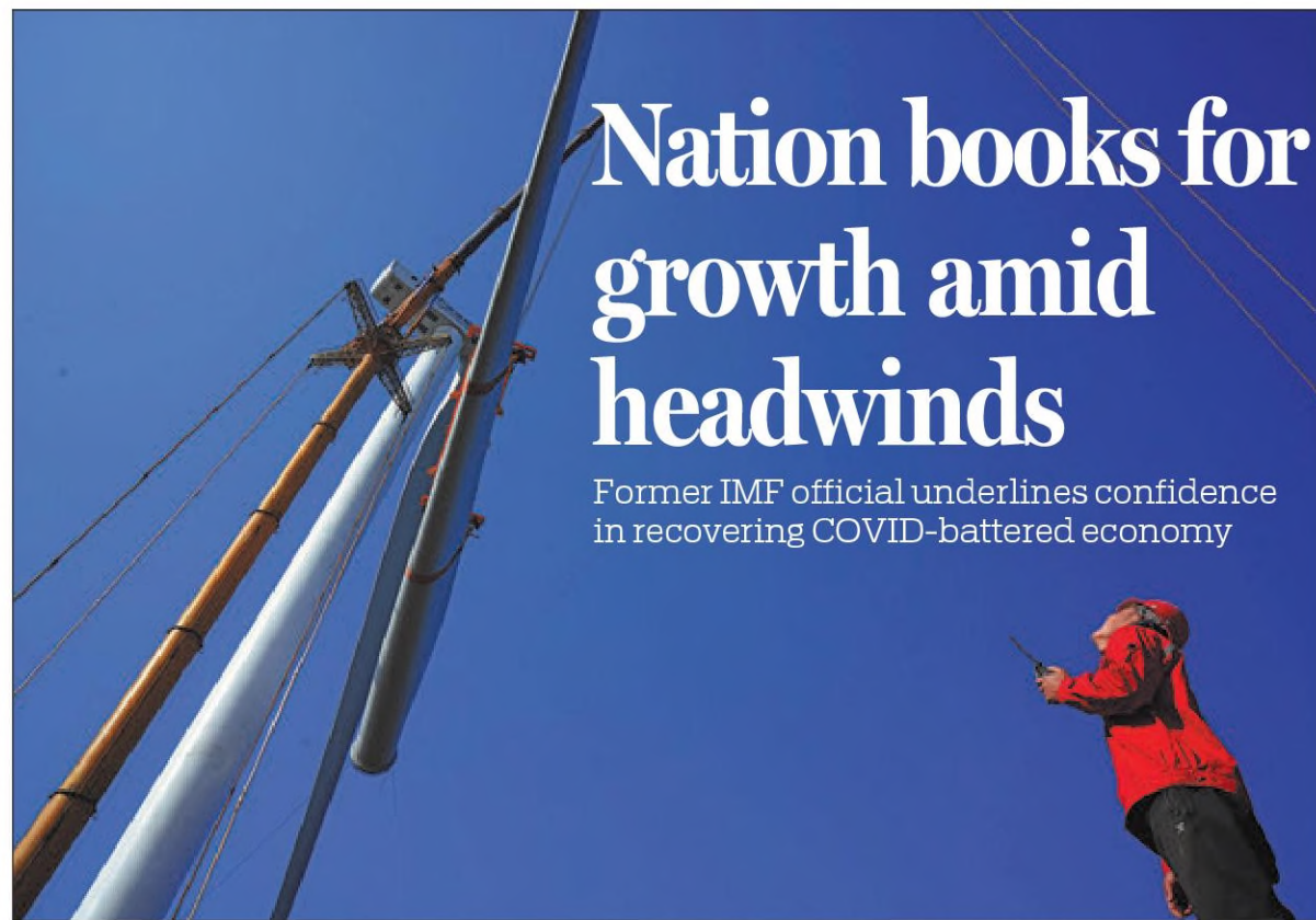
A technician supervises the installation of a wind turbine in Liuzhou, Guangxi Zhuang autonomous region, on Jan 10. LONG TAO / FOR CHINA DAILY
