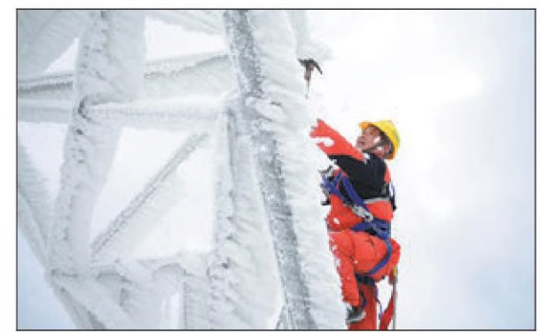
A worker removes snow and ice from a power transmission tower in a mountainous area of Hefeng county, Hubei province, on Tuesday. The local emergency department mobilized a special team to ensure uninterrupted power supply after a cold wave hit the area. YANG SHUNPI / XINHUA
