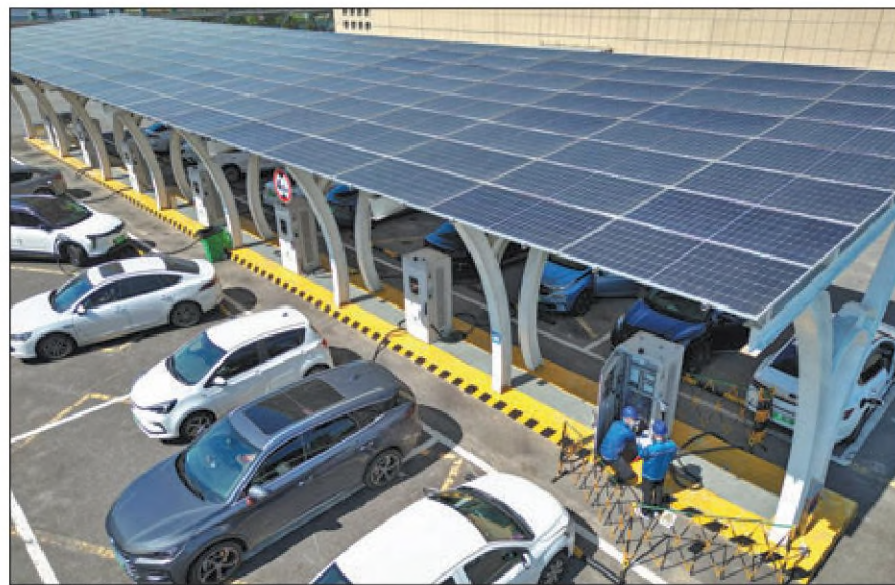
Technicians inspect facilities at a charging station in Yantai, Shandong province, in September. TANG KE / FOR CHINA DAILY
