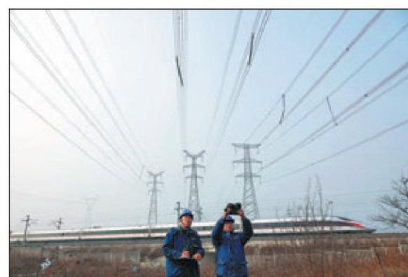
State Grid employees check power lines in Yantai, Shandong province, on Jan 6. TANG KE / FOR CHINA DAILY
