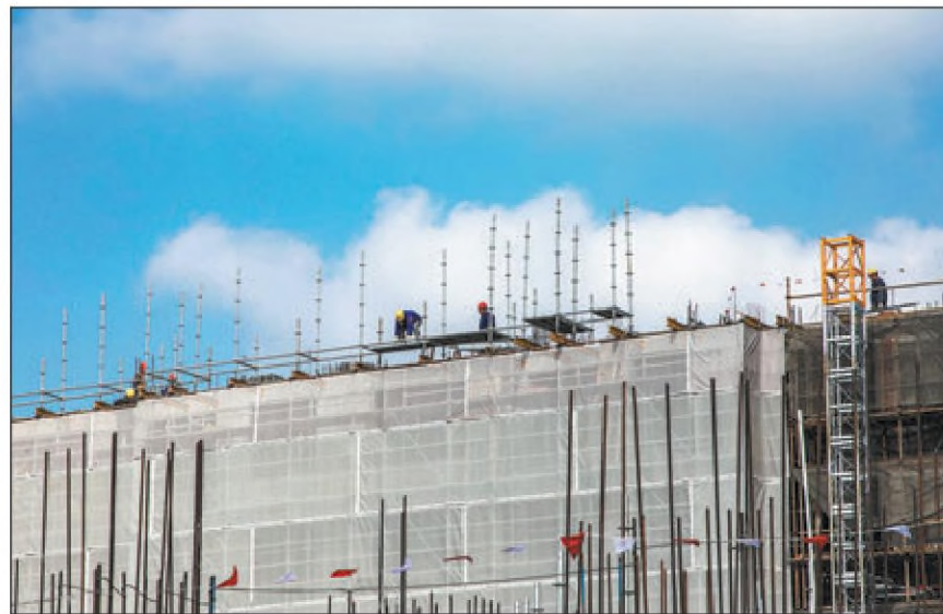
Builders work at the construction site of a housing project in Shanghai on Wednesday. PROVIDED TO CHINA DAILY
