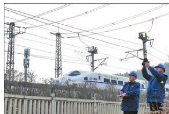
State Grid employees check railway power supply equipment in Yantai, Shandong province. TANG KE / FOR CHINA DAILY
