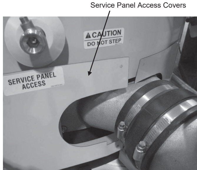
Service Panel Access Covers
