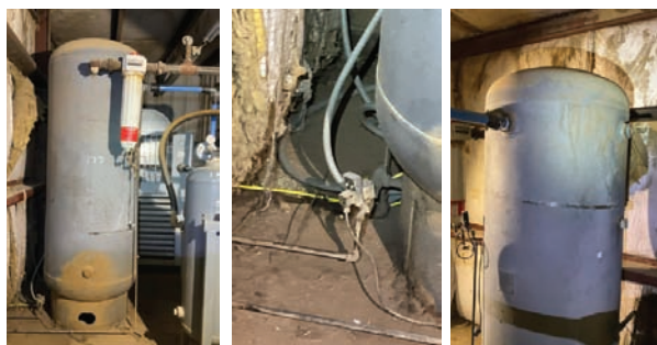
Air Tank Vertical air tank, 34" x 108", electric valve moisture drain.
