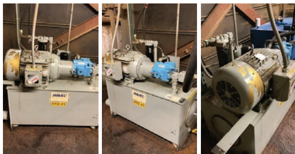
Hydraulic Pack (Part of an entirety) 30 hp electric drive hydraulic pack, 50 GPM, 100 gallon tank, used for optimizing feed system, includes lines to equipment.
