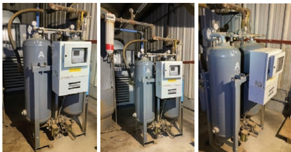
2020 Atlas Copco Air Dryer Model: CD150, SN: APF244452, includes air filters and pipe to tank and to building.
