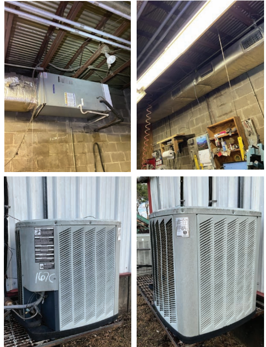
AC Unit Outside and inside units for filing room.
