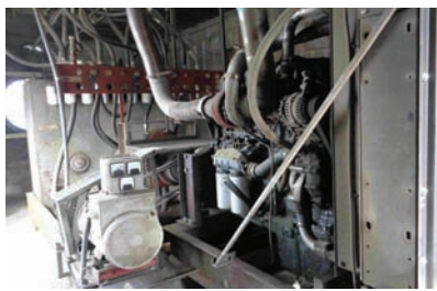
12135A $30,000.00 DETROIT 60 SERIES DIESEL SKID W/600 GAL. HYD.TANK • Power unit skid • 600-gallon oil tank w/oil • Detroit 12.7L 475HP 60 series diesel engine with heavy-duty clutch & hydraulic pumps • 40 KW belt-drive generator. Good well-maintained unit still used daily. All connected hyd. lines and pumps go along with it. Was used to run a Weinig Hydromat H-2000 moulder and various other hyd. equipment. Would sell as a package deal with the moulder. 570-758-2597
