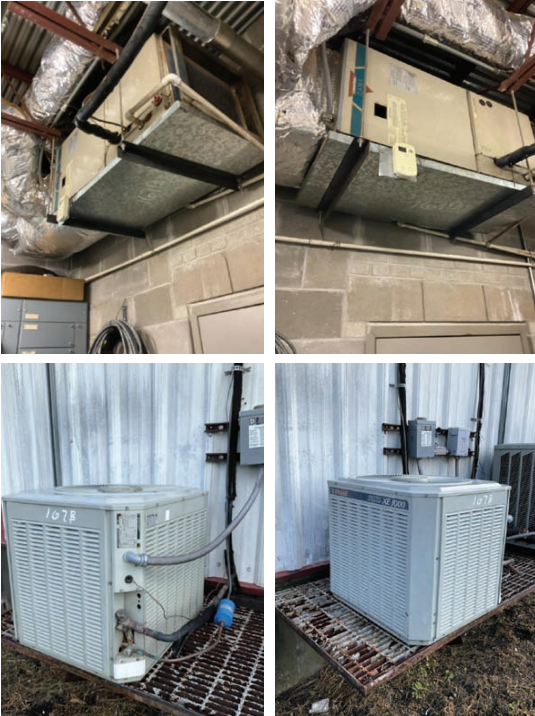
AC Unit Temperature control in electrical room.
