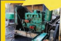
Cummins Power Unit
