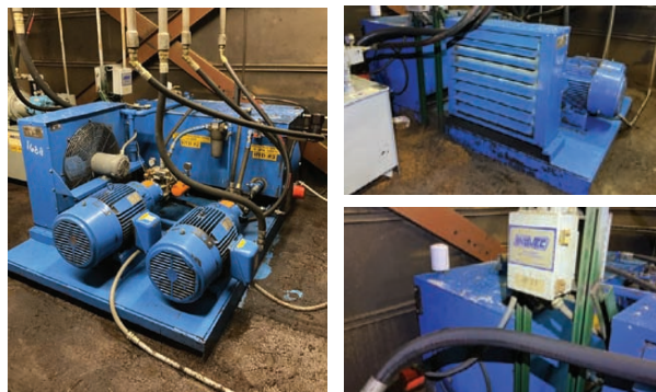
Hydraulic Pack (Part of an entirety) Twin 30 hp electric drive hydraulic pack, edger drive is 34 GPM and roll case drive is 30 GPM.
