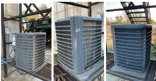
Icor AC Unit Icor international AC unit, includes ductwork on inside of building.
