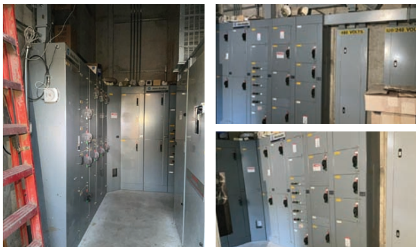
Allen Brady Control Center Rockwell Automation, 16A™ of buckets with starters and misc. electrical for debarker and decks, 2 larger boxes with starters, main breaker and transformer wires to equipment.
