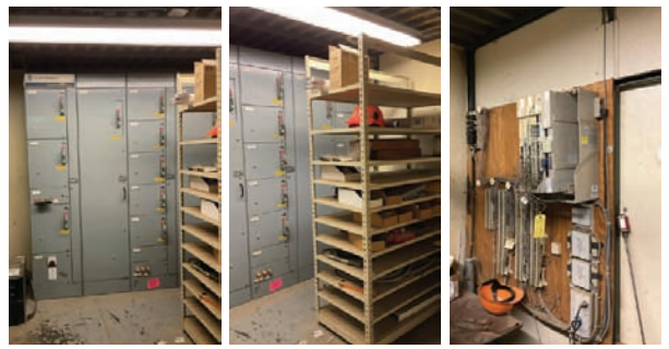
Electrical Room for Edger (Part of an entirety) All electrical in room and wires going to equipment.
