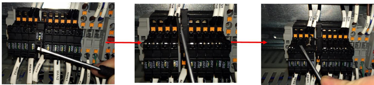
Figure 41: Opening a fuse block
