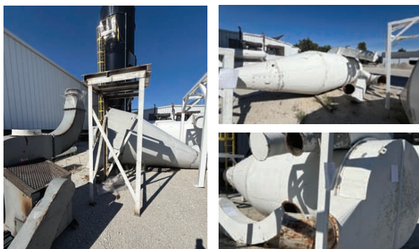
Complete Dust System
