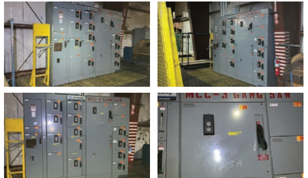
Motor Control Center
