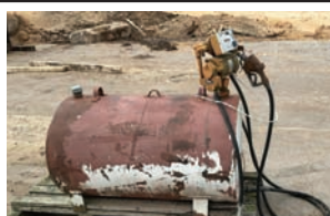
Fuel Tank — Description — Includes Gasboy fuel pump 110v, (condition unknown), Tank: 30" diameter x 49",
