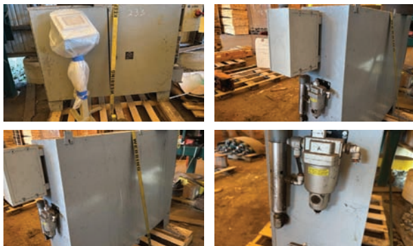
Electrical Control Box — Description — Allen Bradley, with pedestal PanelView Plus 7000
