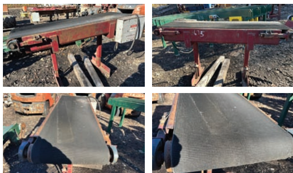
Inclined Belt Conveyor
