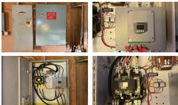
Electric Motor Softstart — Description — 150 hp, cutout box
