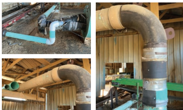
PVC Blower Pipe
