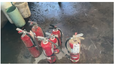
Fire Extinguishers — Description — 6 pieces, 5 good, one needs recharge
