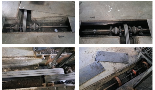
75' Line Shaft — Description — Approximately 75' of 2" line shaft in floor pit connecting to lot#1120 assorted sizes pulleys attached
