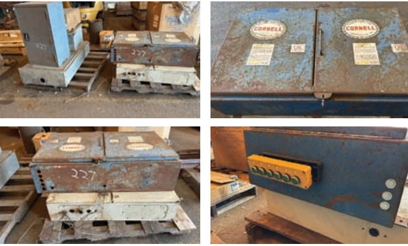
Electrical Boxes — Description — 2 skids, used
