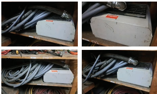
Heater and Electrical Parts — Description — Dayton heater, 480 volt working condition, conduit
