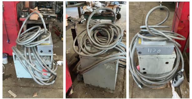
Transformer, Safety Switch, and Conduit — Description — #6 Transformer, Safety switch, unknown length of conduit
