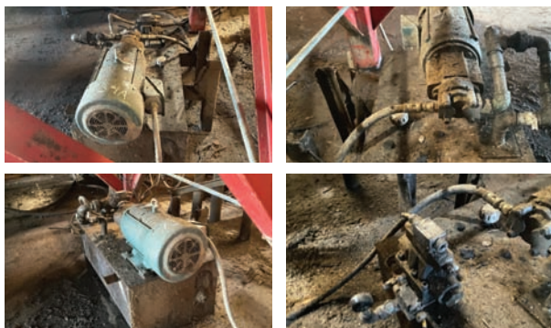
Hyd Pak — Description — 25 hp. Electric motor, solenoid valve that is not being used
