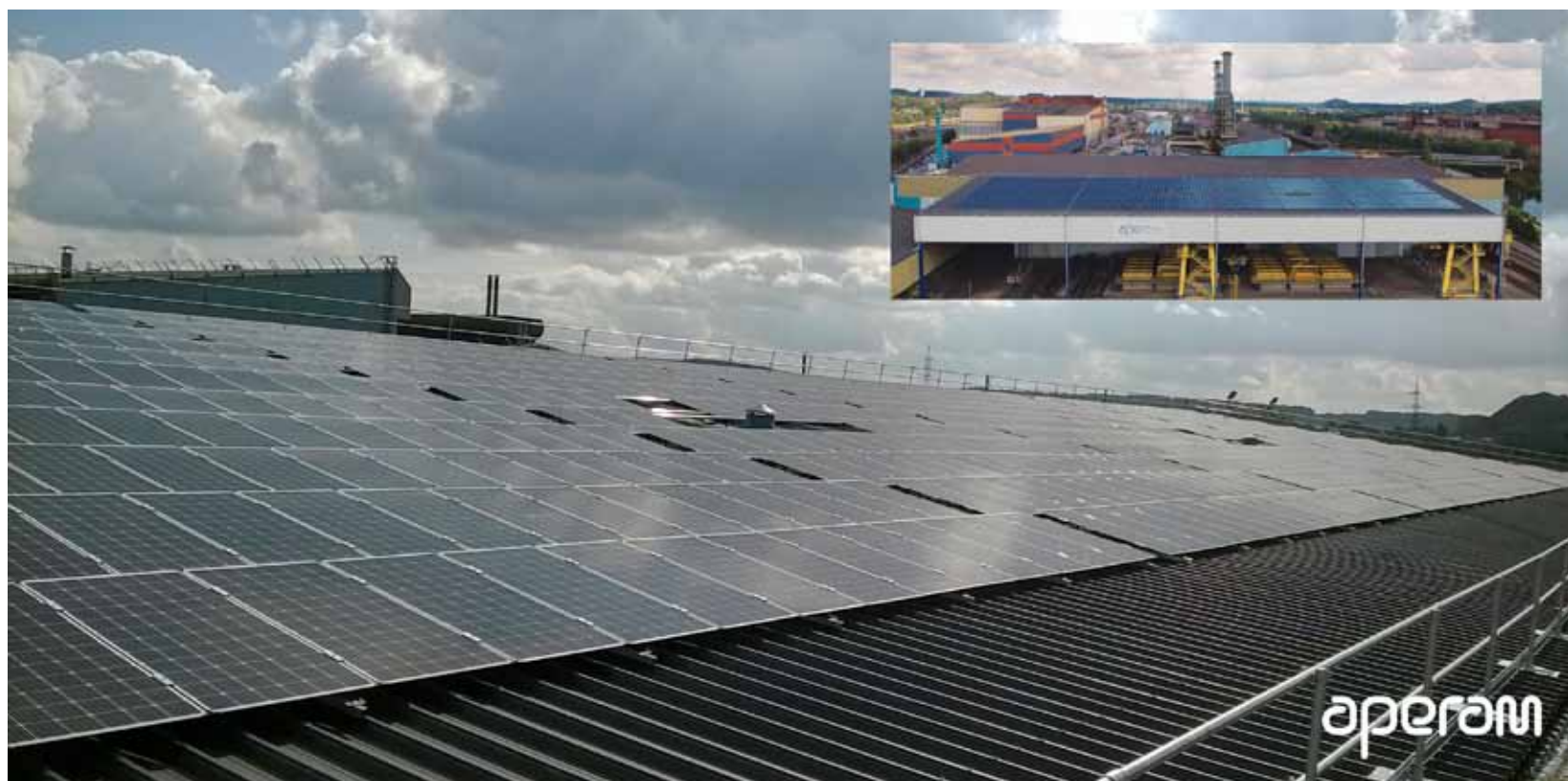
Solar panels installed on Aperam's facility (Châtelet) further demonstrate the company's environmental concerns.
