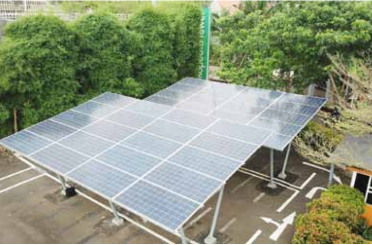
Multipurpose canopy: Tokopedia Tower in South Jakarta has two 13.4-kWp solar canopies that also function as roofs for its parking lots.
