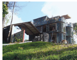
1 In Bocas del Toro, Panama, an ecoresidential community called Plastic Bottle Village uses its namesake for building insulation.
