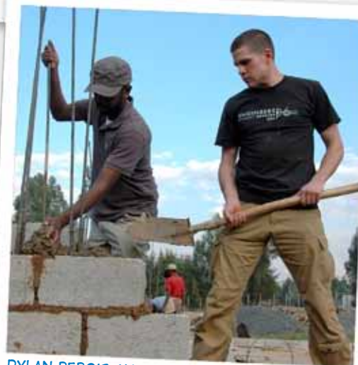
DYLAN REBOIS AND ENGINEER DANIEL ENGIDASHET BUILD A REINFORCED MASONRY COLUMN FOR THE YOUTH CENTER IN ADDIS ALEM, ETHIOPIA (EWB-U MARYLAND)
