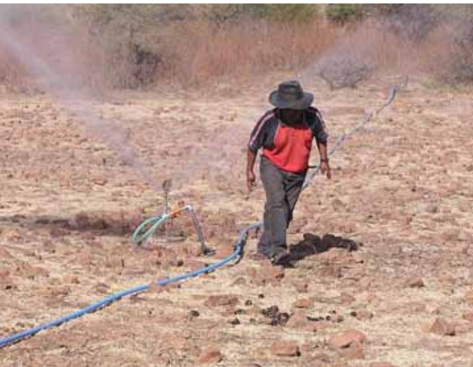
In July 2007, EWB-USA University of Washington chapter tests the new irrigation system they installed. Testing the system is the town leader, German Condori. (Photo by University of Washington)
