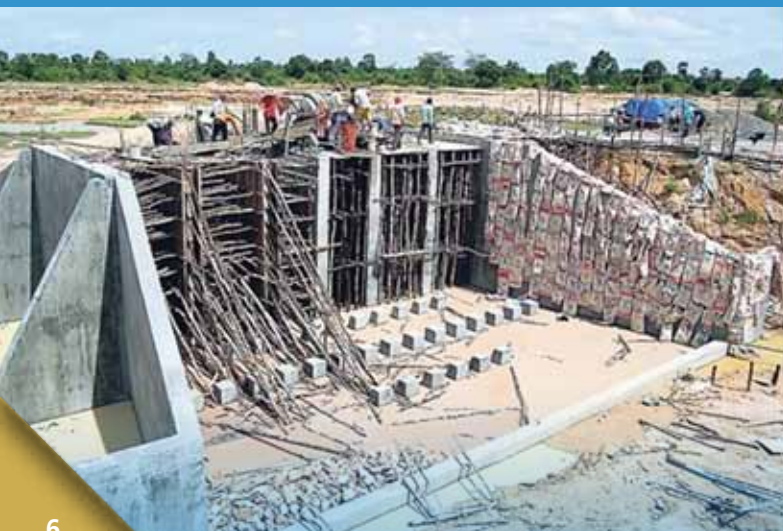
Cambodia Water Dam Project to place a watergate for the Balang Commune. This project serves at least 18,000 people. This project utilized too many volunteers to list and we averaged three to four site visits a year. (New York Professional Chapter)
