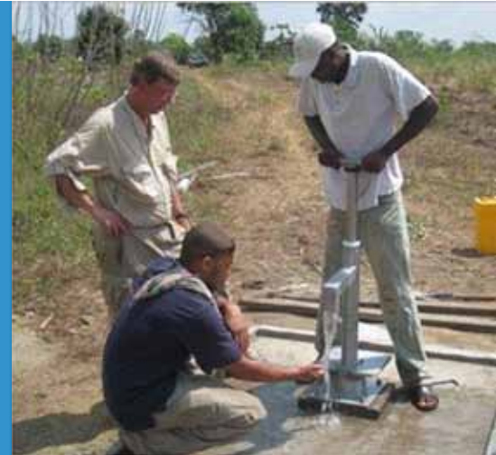
EWB-USA Las Vegas Professionals Mike Sheffer and Anthony Deleon watch while a member of the volunteer labor force from Tsito Awudome, Volta Region, Ghana primes the hand pump well that was installed during their February 2009 trip. (Photo credit to Kosi Yinkah, director of DIVOG, local Ghana NGO).
