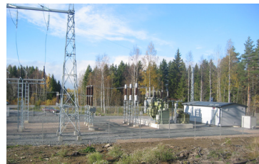
Distribution substations With 100 years experience, the world leader in turnkey air and gas insulated substations
