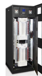
Cyberex® from Thomas & Betts Products include digital static transfer switches, power distribution units, remote power panels and UPS
