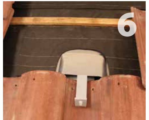
6 Flashing must be sealed to deck using three-course method with mastic and mesh, see page 2, or underlayment bibbing. When bibbing, the upper edge of the bib should extend 3" under the course of underlayment above the flashing and the bib should be wide enough to overlap the sides of the flashing by 3".
