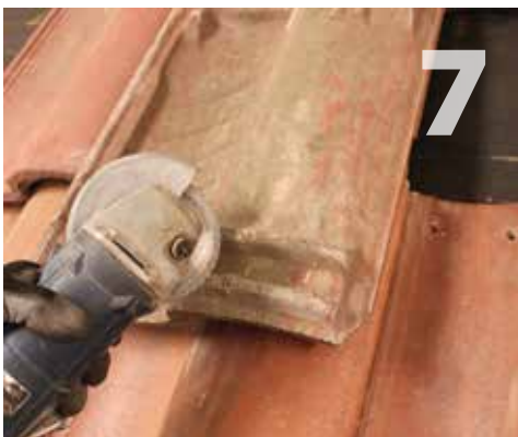
7 Cut a clearance notch in the weather guard lug using a grinder with tuck point blade. Make sure the tile seats back down in it's original position. Leave at least 1/4" of tile to prevent breaking through.
