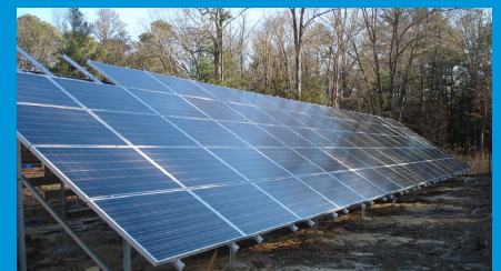
18 kW New Jersey PLM-P235 modules
