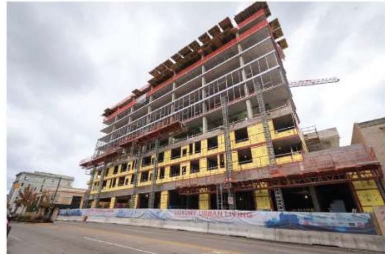
Mixed-income housing project with 45 market rate units and 45 units for low income earners.
