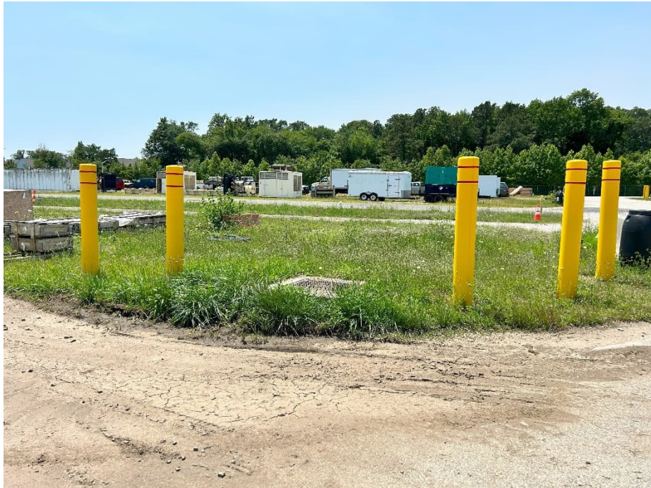
Photograph 23. View of storm drain with grass and sediment; a sediment filter sock is in place.
