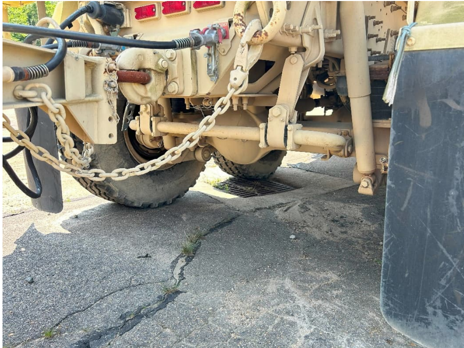
Photograph 21. Sediment accumulation around storm drain in central area of the OU.
