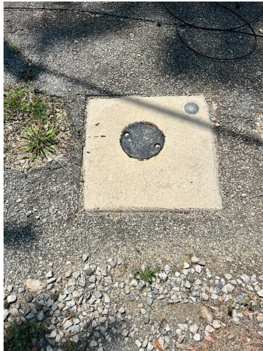
Photograph 4. Typical flush mount monitoring well at OU 3.
