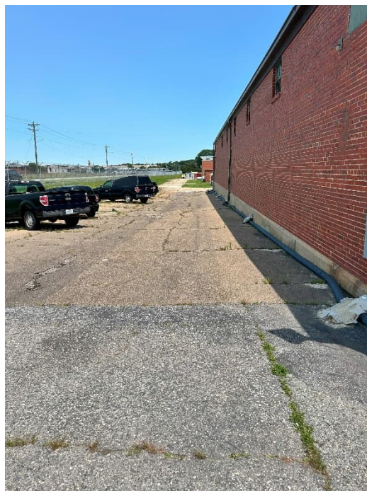
Photograph 2. Deteriorating asphalt west of Bldg. 153.
