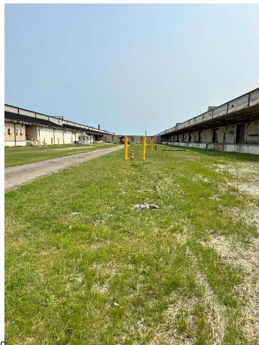
Photograph 20. Depression near storm sewer and water line between Bldgs. 65 and 66.
