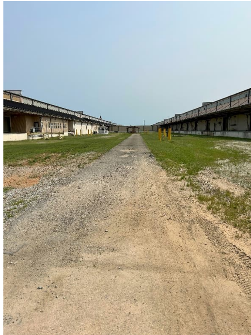
Photograph 13. Deteriorating pavement on access road between Bldgs. 65 and 66.
