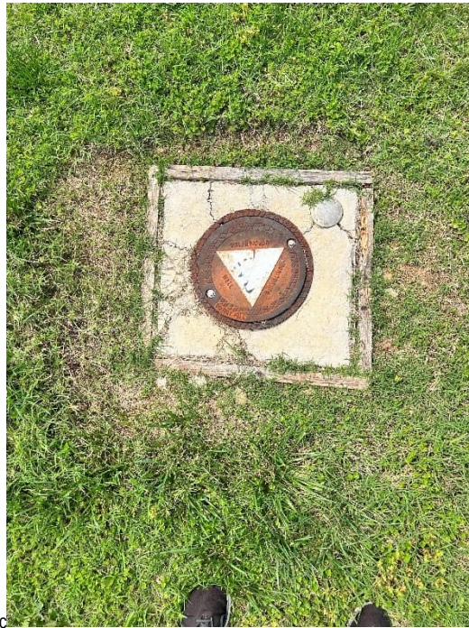
Photograph 21. Flush mount well completion, concrete cracked from equipment passing over.
