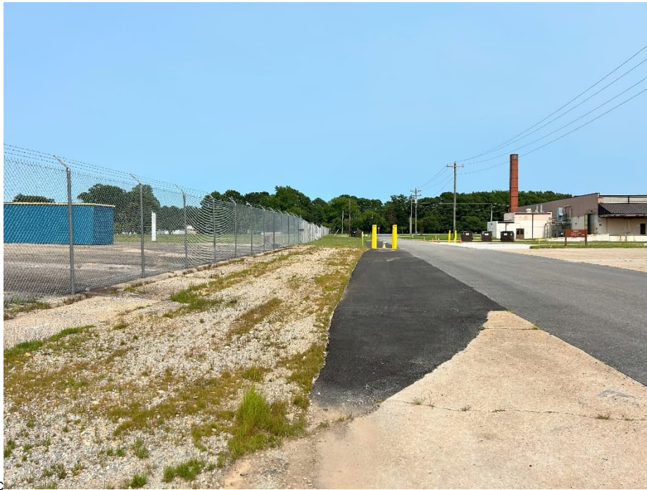
Photograph 29. Repaved area north of Bldg. 65, MW-119 destroyed during construction.
