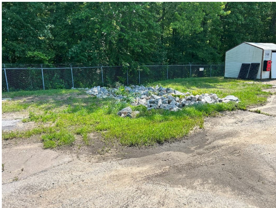
Photograph 18. View of rip rap run off area collecting sand and gravel.
