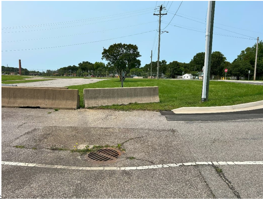
Photograph 17. View of storm drain where southern pump test discharged, cracking in asphalt visible.
