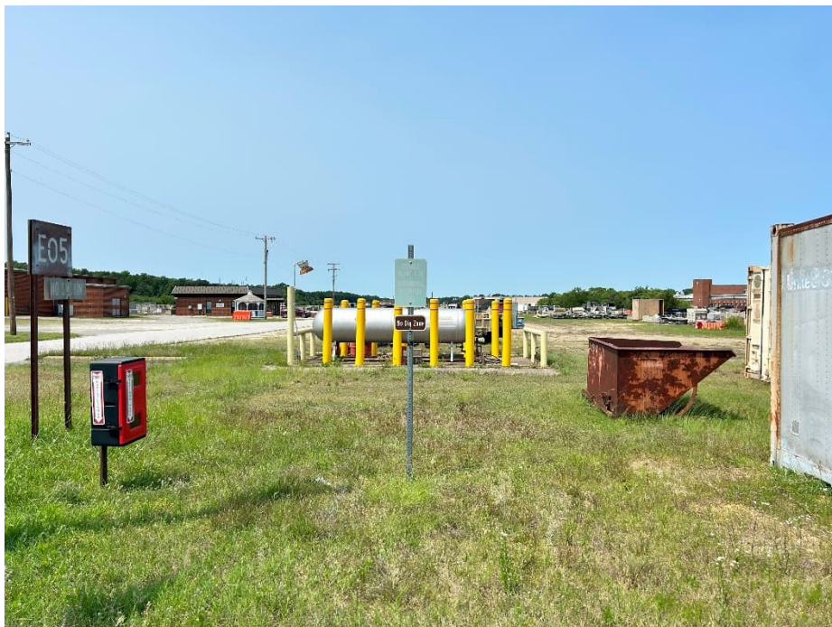
Photograph 6. View of propane fuel tank east of Bldg. 40.
