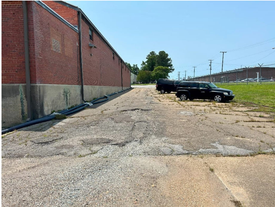
Photograph 19. Southward view of western side of Bldg. 153 showing cracked asphalt.
