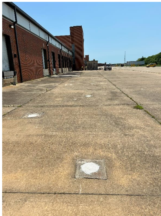
Photograph 8. View of typical flush mount well, abandoned during monitoring network optimization activity.
