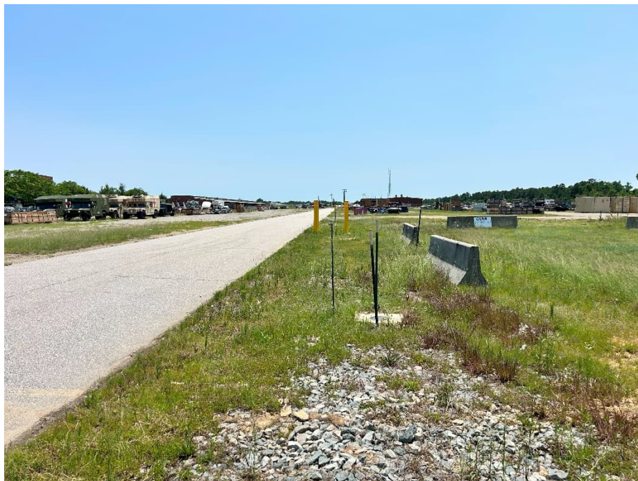
Photograph 22. Depression following the water line in the open storage area.
