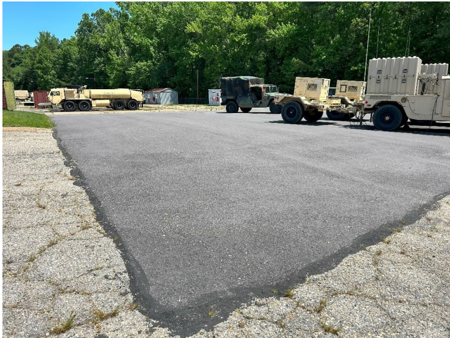
Photograph 20. View of southern asphalt repair area from southeast corner of Bldg. 150.
