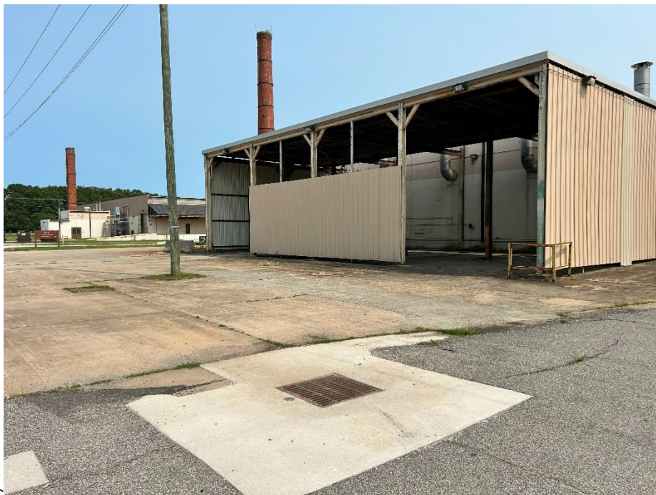
Photograph 16. View of exterior of covered storage area, showing cracking asphalt at storm sewer repair area, completed FY24.
