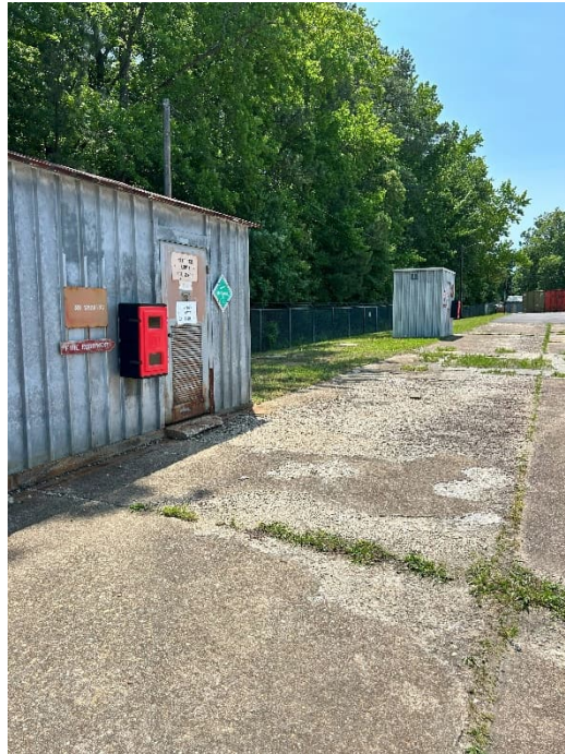
Photograph 17. Looking south along wooden fence line, showing deteriorating concrete.
