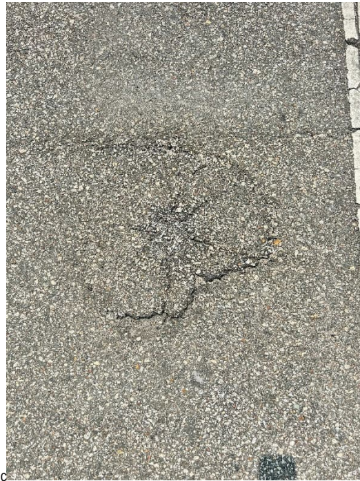
Photograph 19. Asphalt patch at 2022 injection location in the Bldg. 66 area.
