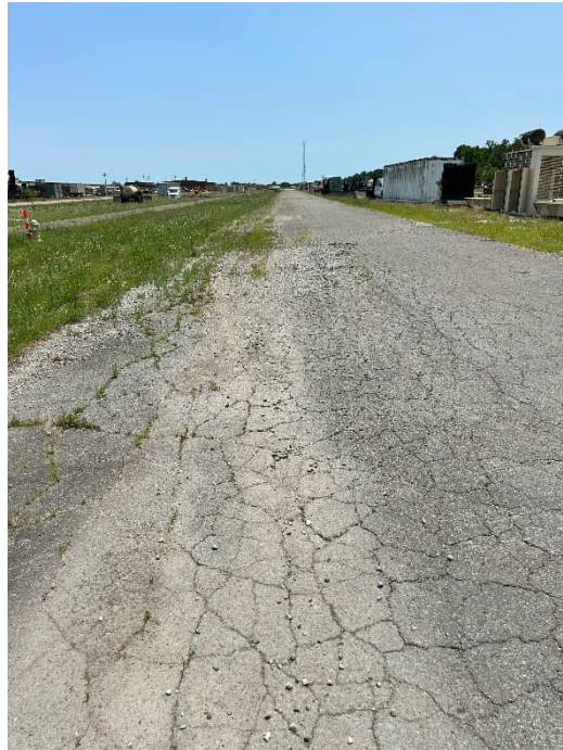
Photograph 29. Looking south from northern end of OU 1, showing asphalt deterioration in open storage area.
