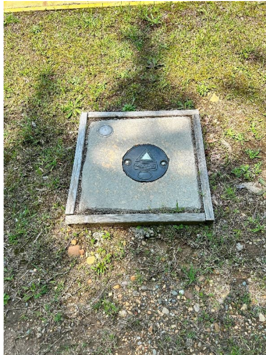
Photograph 15. Typical flush mount monitoring well completion in grass, installed 2021.
