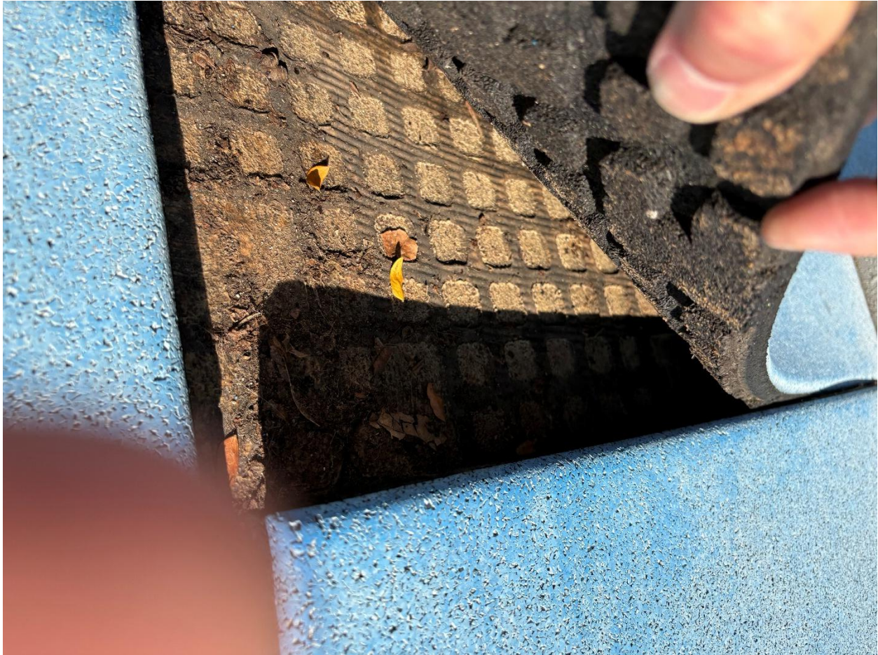
Closer picture view of the same tile where there is little to no bond of the adhesive to the back of the tile.
