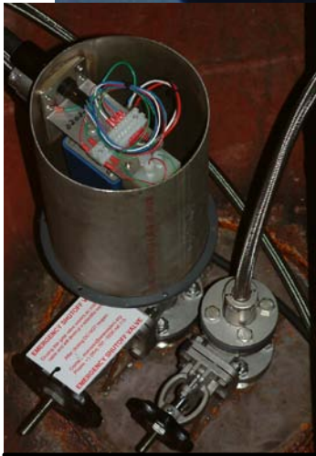
Inflow & Outflow Valves
