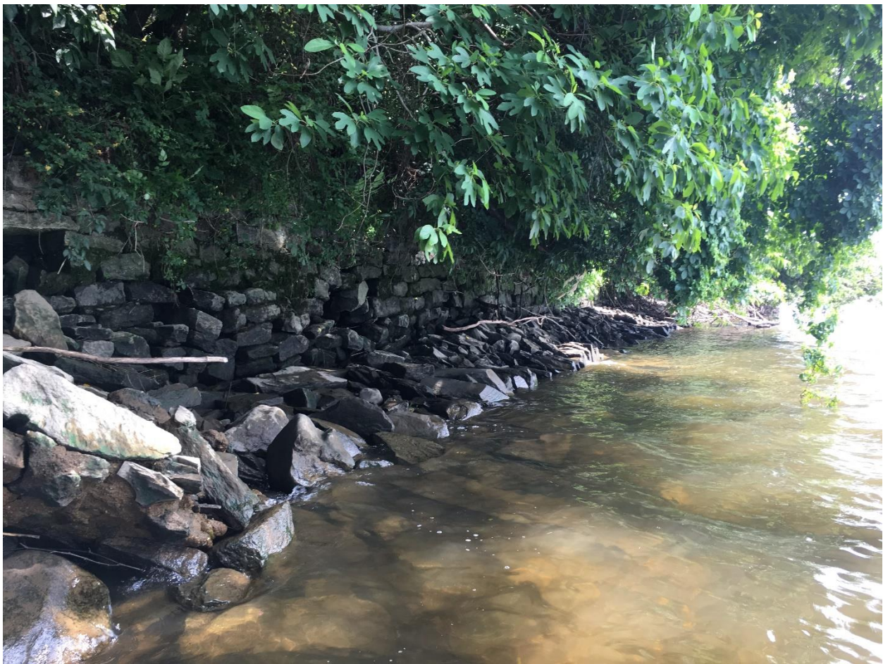
Figure 15. Glen Foerd on the Delaware north of the gazebo looking at a hardened shoreline with rip rap and an old retaining wall
