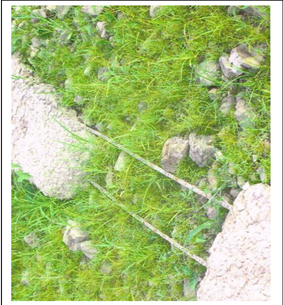
Left: Detail of rebar connection. The photo has been rotated left 90°. Allyn Lord photo
