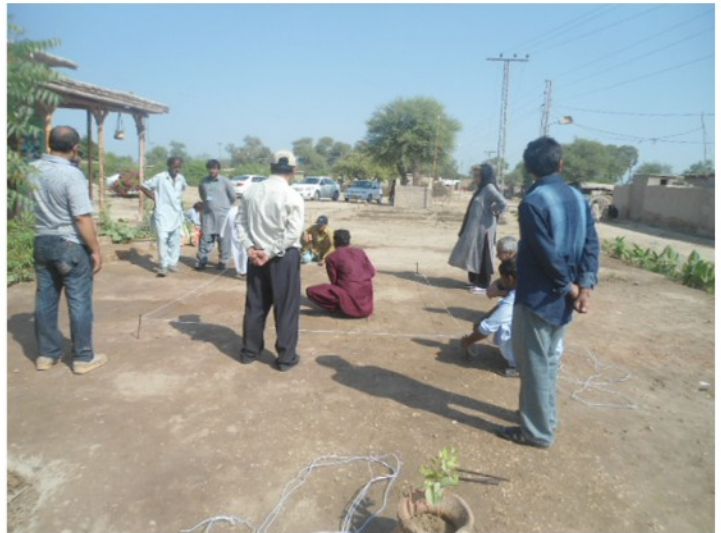
The participants marking a layout for a room. Mr. Naheem Shah and Engr. Shahjahan Khuwaja providing directions.
