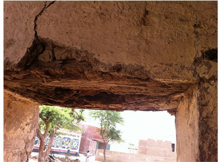
Damaged lintel in the veranda
