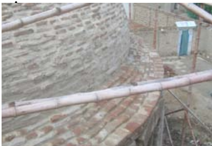
The underpinning of the top of the wall protected against rain water.
