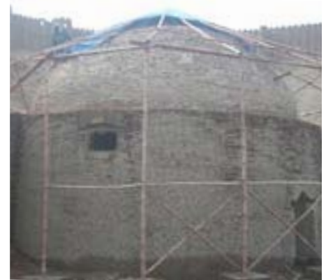
Granary 5.3 after heavy rains.
