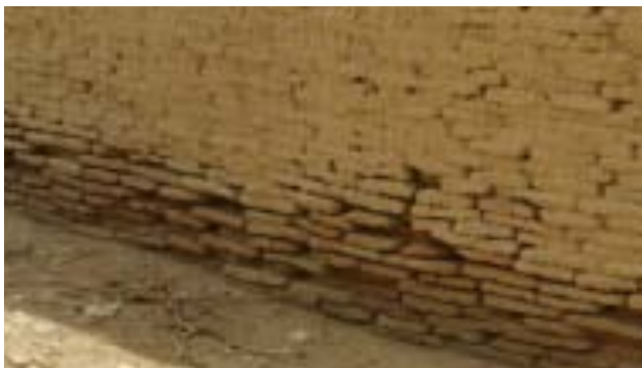
Work on external wall will require underpinning, filling of joints with new mortar and providing plinth protection / toe arrangement with lime render to provide protection from rain water to the base of external masonry wall.
