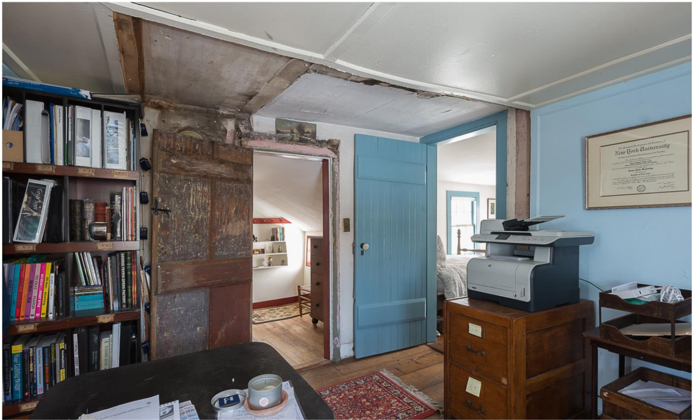
Photo 23. Interior view southwest showing doorway to southeast bedroom and doorway to northwest bedroom from northeast room on second floor.
