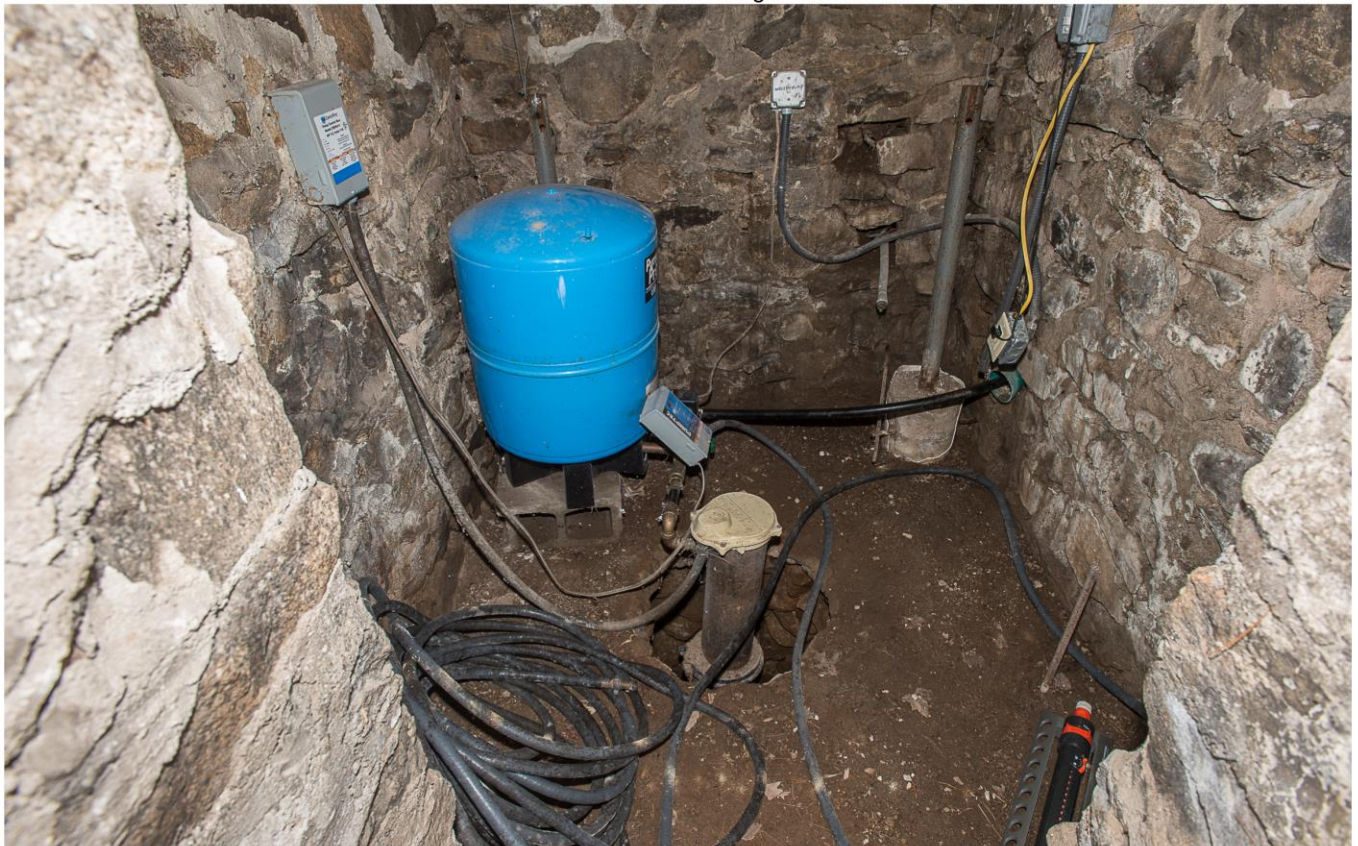
Photo 10. View north showing well house interior.
