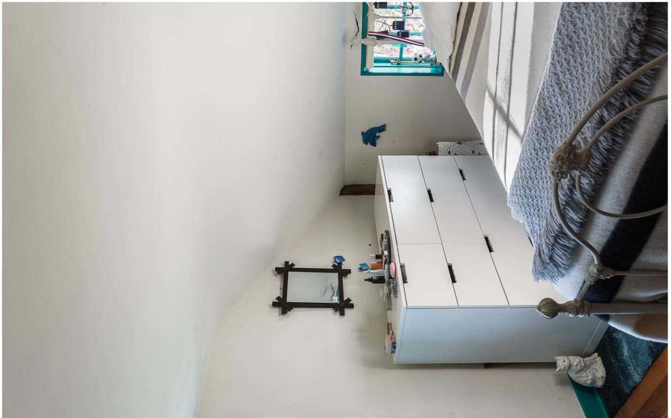
Photo 24. Interior view southwest showing southwest corner of southeast bedroom on second floor.
