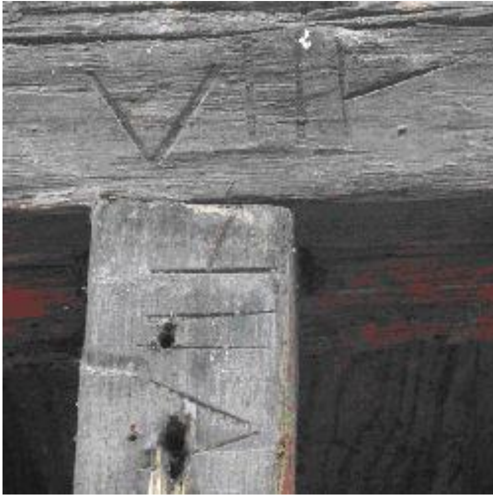
Figure 4. Characteristic marks used in scribe rule framing. (Connecticut Trust for Historic Preservation)
