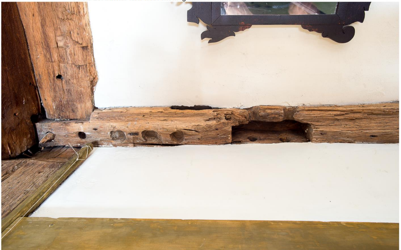
Photo 26. Interior view northwest showing unused mortises in timber frame on second floor.
