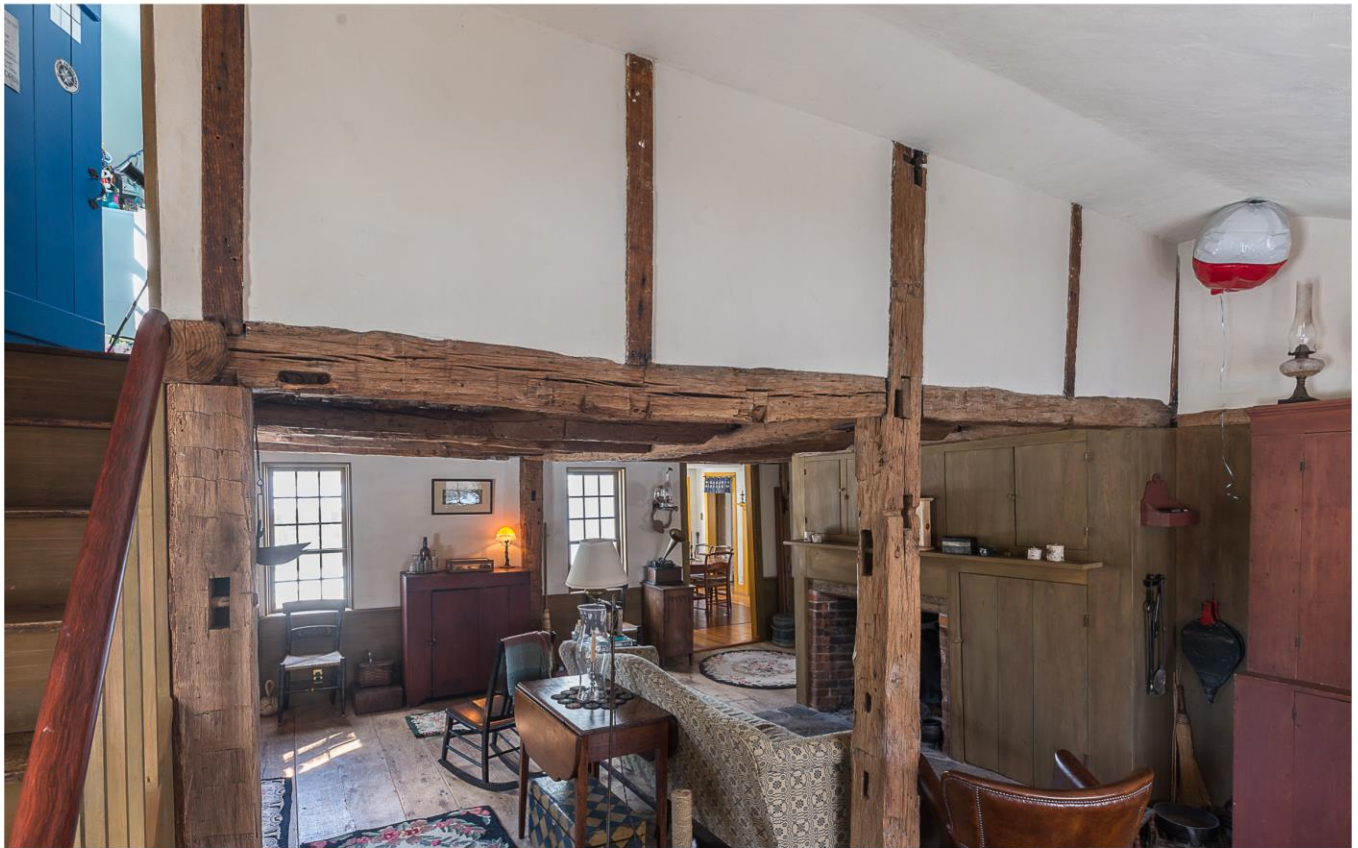
Photo 25. Interior view west showing unused mortises in timber frame on first floor.
