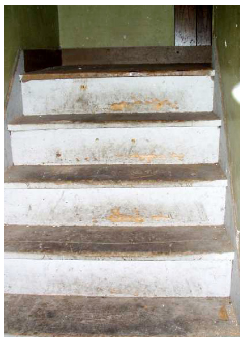
FIGURE 5.6a Friction hazard on stairs pre-treatment.
