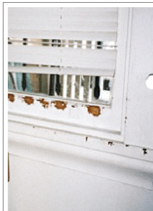
FIGURE 5.8 Chewable surface: teeth marks on window sill.
