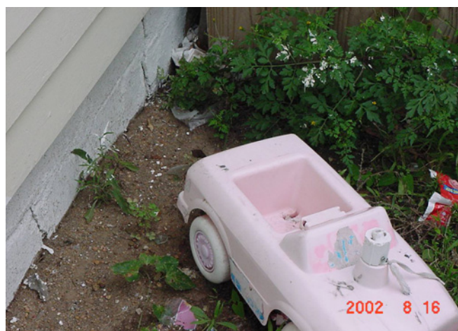
FIGURE 5.9 Soil lead hazard at dripline
