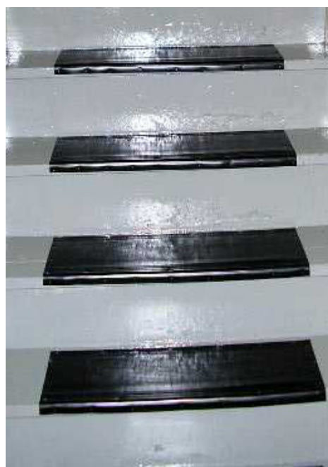
FIGURE 5.6b Friction hazard on stairs post-treatment.
