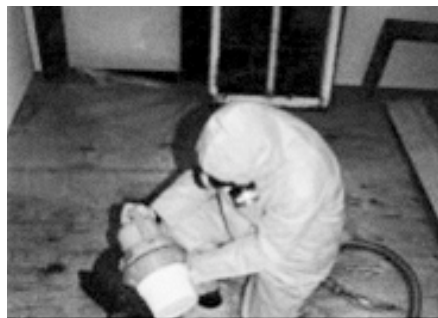
e) Wash/Replace Coarse Prefilters if Necessary
