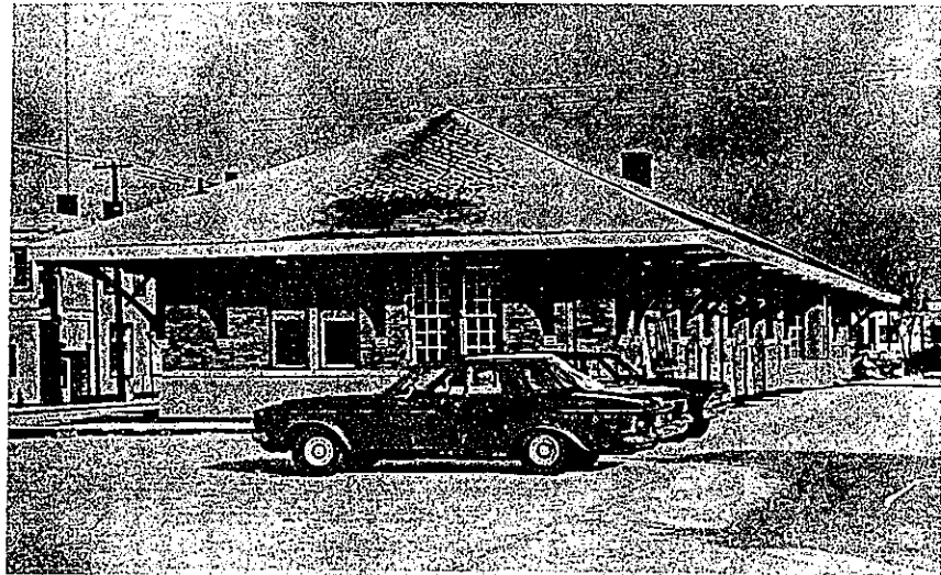
Exterior of the Timmins station has taken on a bright new look. The brick has been sandblasted. New windows will also be installed.
