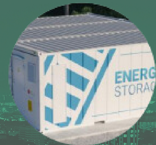
(BESS) Battery Energy Storage System
