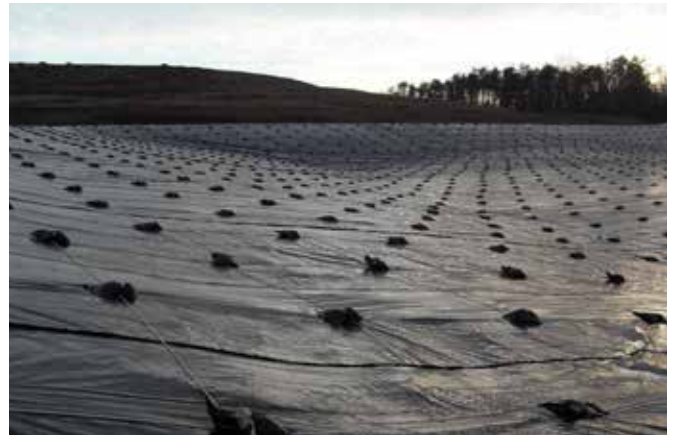
Landfill Odor Control Barrier Cover
