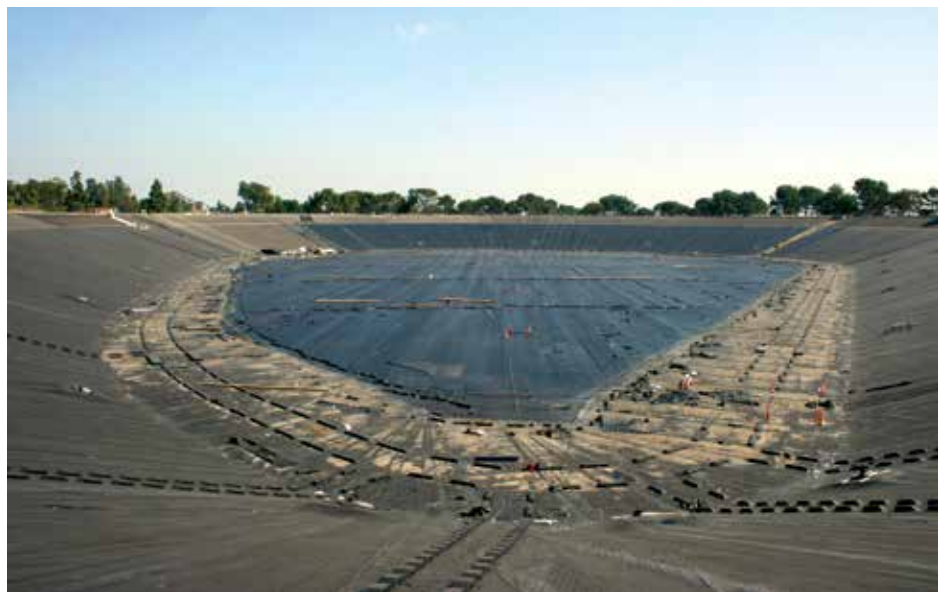
FIGURE 5 Cover installation at 90% with perimeter rain collection trough (RCT) and radial RCT
