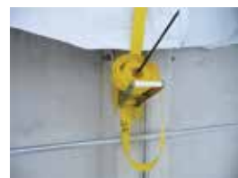
Photo 6 – Webbing tied to wall
